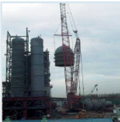
Upper Part of Regenerator
