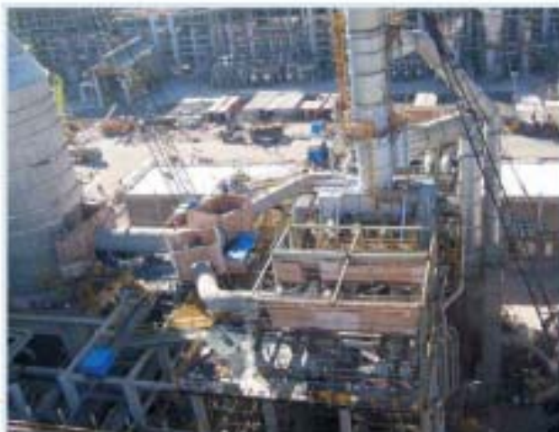
Overall View of Reliance VDU
