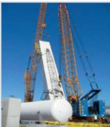
Cold Box on installation
