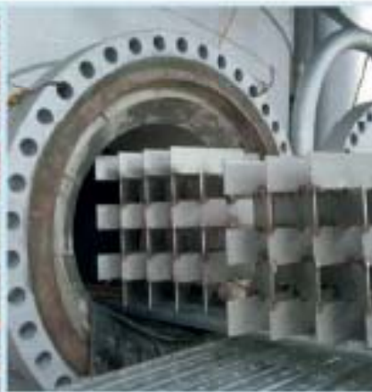
RX Stripper Packing on Install.
