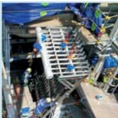
New Coil on Installation
