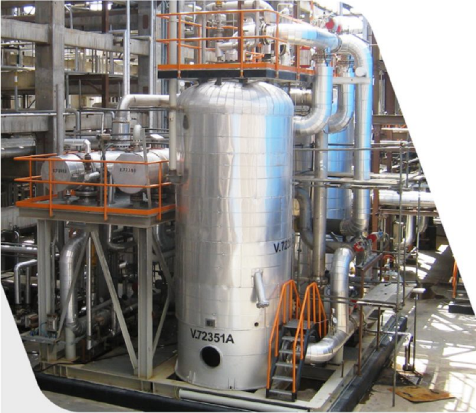
Isfahan Refinery Gas Dryer
