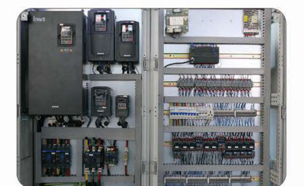
电器操控系统 Electric control system
