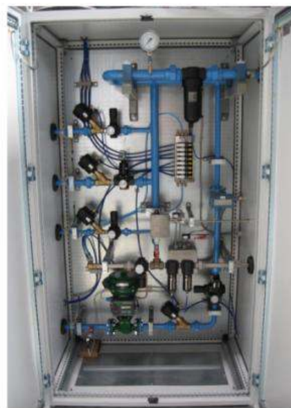
Pneumatic cabinet 气动控制柜
