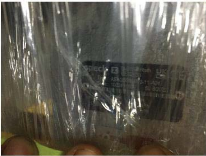
During nameplate check of the oil pump op1
