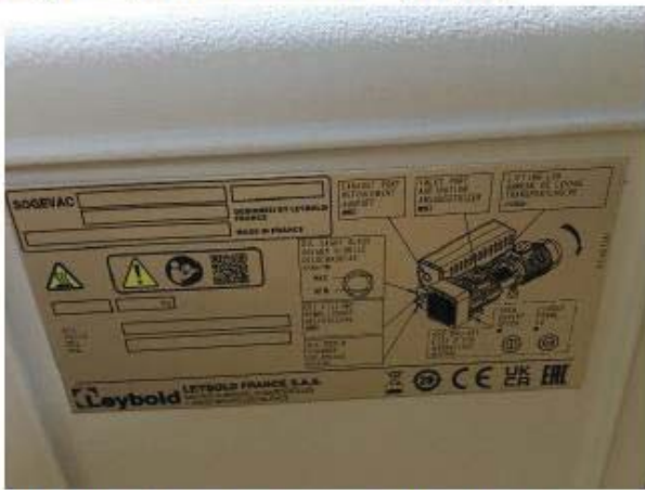
uring nameplate check of the vacuum pump
