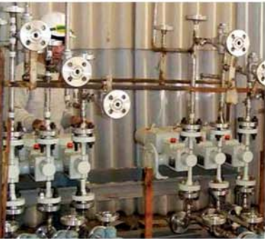
Plant South Pars Phase 4 Offshore EPC SADRA Item Chemical Injection Package Material CS/Inconel 625 QTY 6
