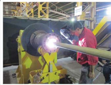
Weld Overlay : Internal of Pipe Column & Boom Internal Pipe Cladding (min ID: 4 in - max length each side: 1 m) Weld Overlay
