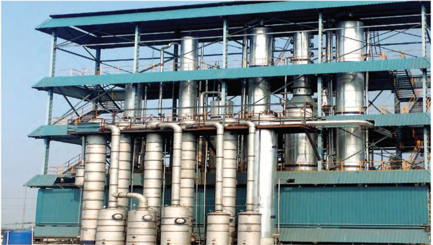
Integrated Evaporation Plant for Bio-methanated Spent Wash on Multi-pressure Distillery
