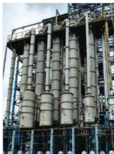
Hybrid Evaporation Plant for Bio-methanated Spent Wash
