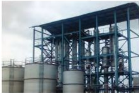
Evaporation plant for Bio-methanated Spent Wash
