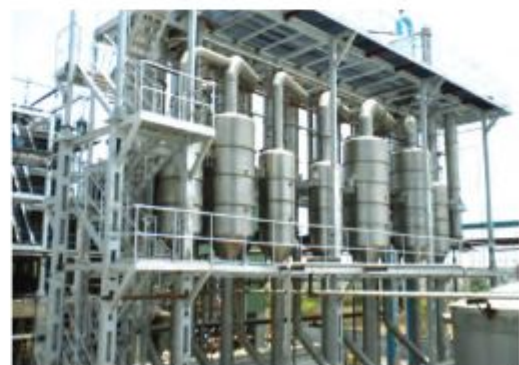
Evaporation plant for Grain based Distillery
