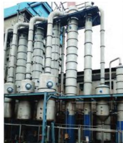
Hybrid Evaporation Plant for Bio-methanated Spent Wash
