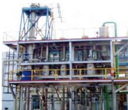
Zero Liquid Discharge Plant for Pharma Industry
