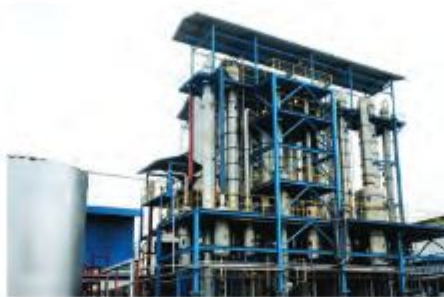
Evaporation plant for Raw Spent Wash
