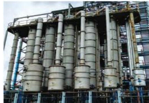
Evaporation Plant for Bio-methanated Spent Wash
