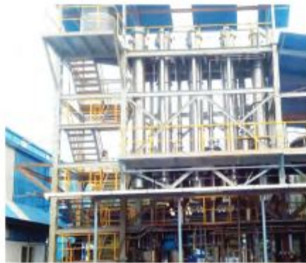
Zero Liquid Discharge Plant for Specialized Tile Manufacturing Industry
