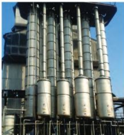
Integrated Evaporation Plant for Raw Spent Wash
