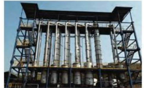
Evaporation plant for Bio-methanated Spent Wash
