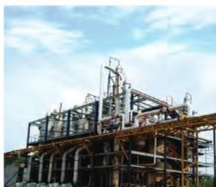
Zero Liquid Discharge Plant for Palm Oil Industry
