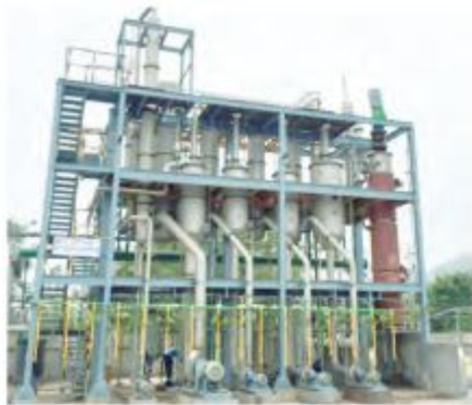
Zero Liquid Discharge Plant for Common Effluent treatment Plant (CETP)
