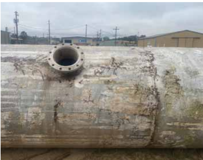
⌚ Vertical NEN style turpentine condenser with stress corrosion cracking (before repair).
