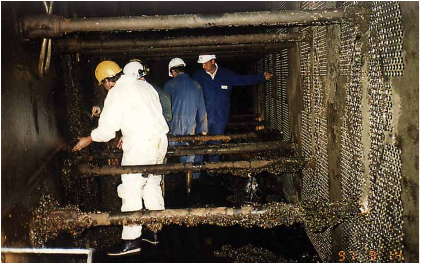
⚡ Inspection of heavily fouled water inlets and condenser tubes at a power plant.
