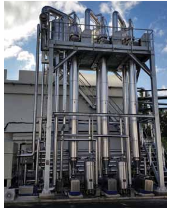
➤ HRS has installed ZLD systems for clients in Europe. Image courtesy of HRS Heat Exchangers.
