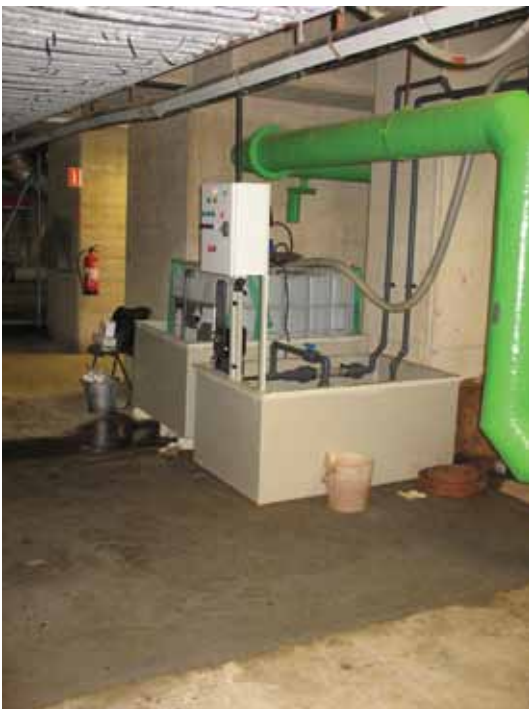
➤ An example of a typical injection system suitable for Blueterm® used at a power plant in the Netherlands.
