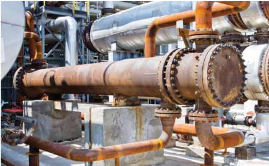
➤ New but not yet painted mounted heat exchanger is connected to piping in a plant for refining.
