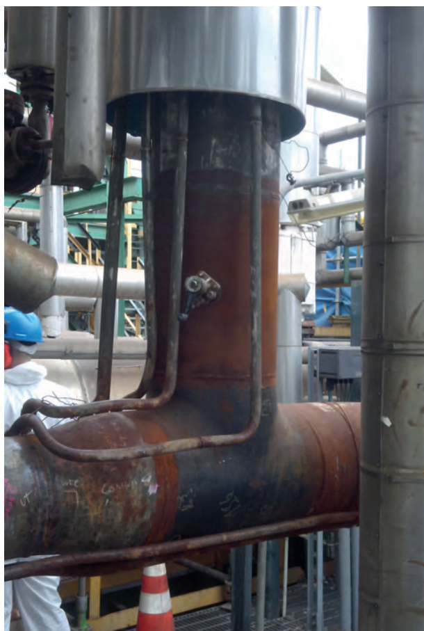
Figure 2. URA2 tail gas piping tracing.
