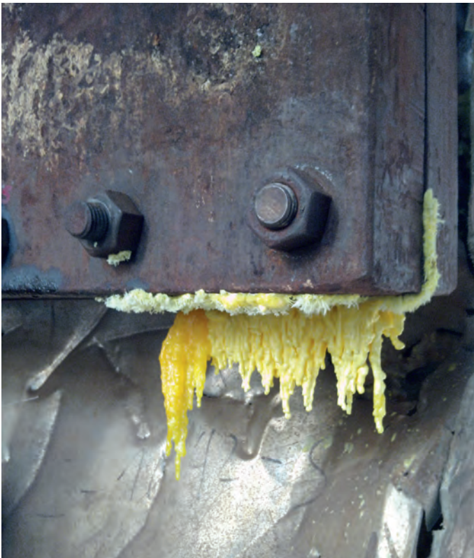
Figure 5. Evidence of sulfur from the demister box in URA2 Third Condenser C-1644.
