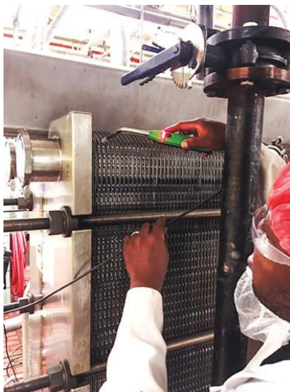
IMAGE 1: A precision sensor is used to detect the discharge of any gas and to signal damage to the plate or gasket. (Images courtesy of Rodem)
