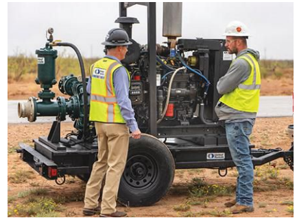
IMAGE 2: When it comes to construction site dewatering, there is a lot riding on proper pump selection.
