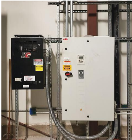
IMAGE 1: Variable frequency drive (Images courtesy of EDE Electric Motor Testing)
