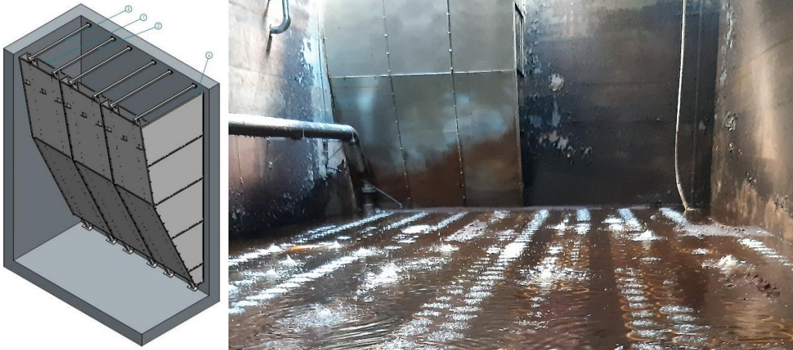
Figure 9: Drawing of DEMON baffle wall with three elements (left) and installation in the reactor (right).
