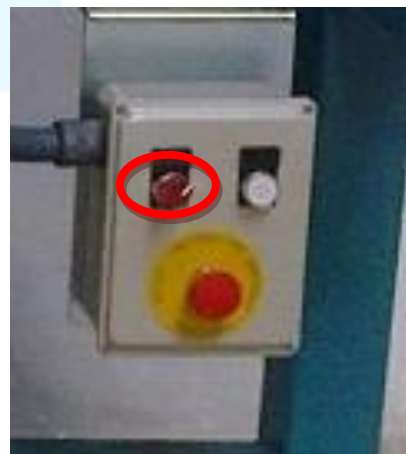
Unloading cabinet loading permission switch
