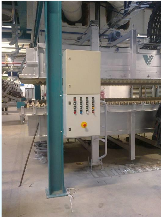
Tempering control cabinet
