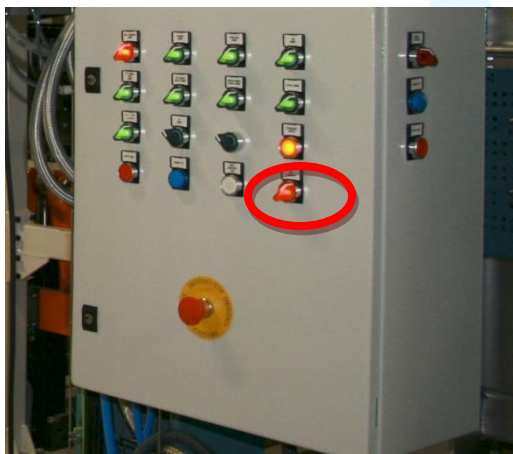
Tempering cabinet loading permission switch
