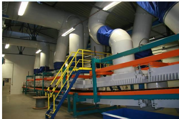
Cooler conveyors view
