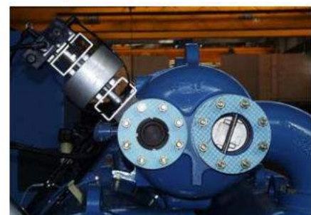
Fig. 17: By-pass valve and check valve
