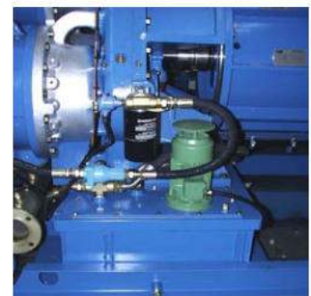
Fig. 23: Pre/post lube oil pump
